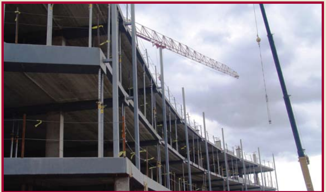
The Bridgeview is a mixed-use complex in Chattanooga, TN, constructed in 2008 using the DIVERSAKORE framing system throughout. “Speed, simplicity and cost savings were the major benefits to the developer,” explains President Marc Rahimzadeh. “We were able to bring efficiencies and savings throughout the project, including labor. The lower beam profile minimizes total building height, which means less exterior exposure and thus lower skin costs.”
