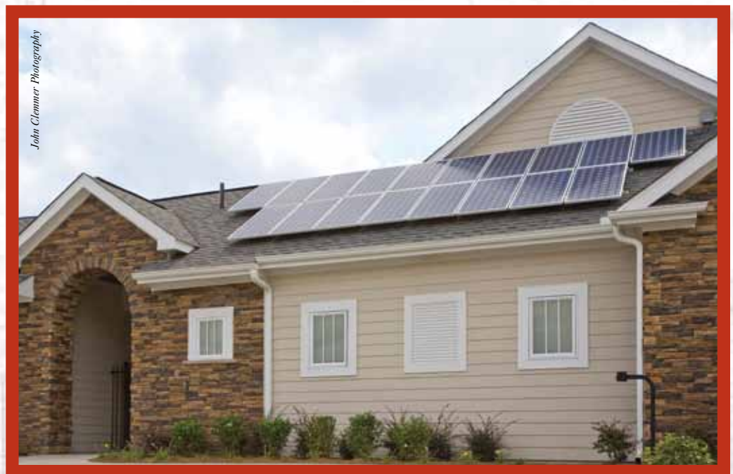
Ansley at Princeton Lakes features solar panels on their clubhouse. “The company’s philosophy has always been to be ahead of the curve when it comes to things like green building,” explains Senior Project Manager and LEED AP Trip Booker. “We’ve always tried to minimize our impact on the environment, even when it costs us a bit more. It’s just the right thing to do.”
